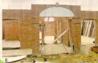
A Carlos Itano, a carpenter for Chateau Constructions works on the house, which is reaching completion
